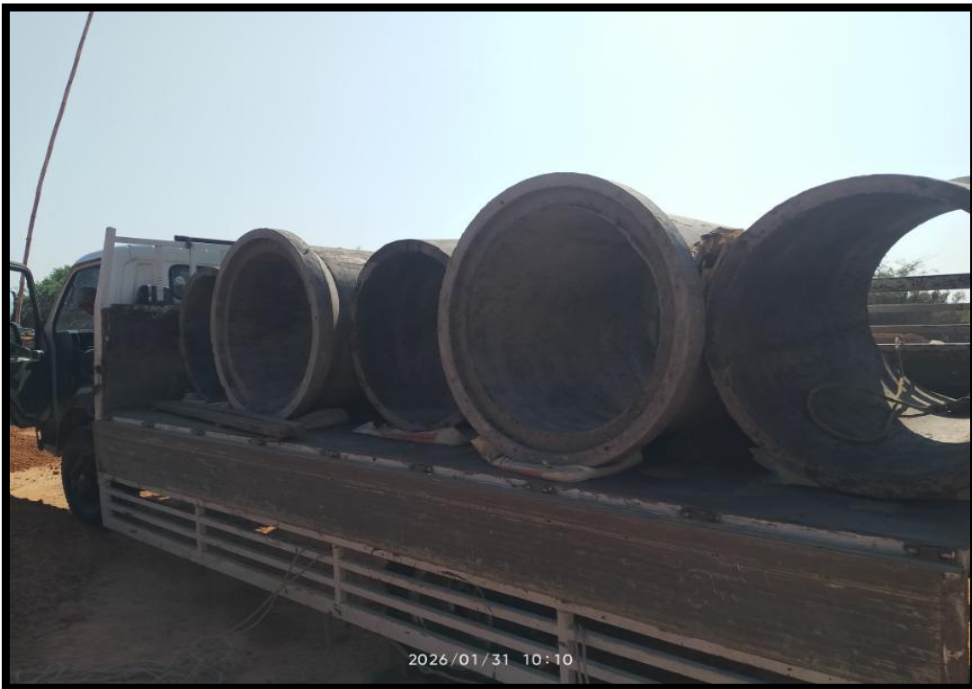
Item : Concrete Water Pipe Delivery work Description : Temporary Diversion Water way Date Taken : January 31, 2026
