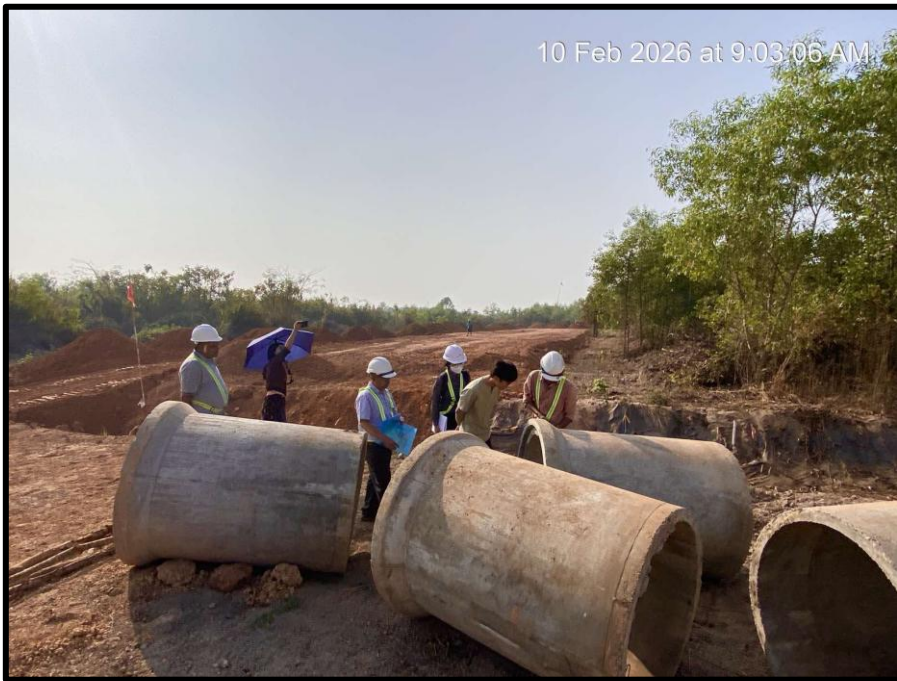
Item : Site Inspection by KMIC Description : Testing R.C.C Concrete Pipe Date Taken : February 10, 2026
